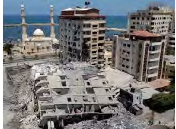
Buildings used by Hamas leaders to hide or meet were high value targets for the IDF surgical attacks
